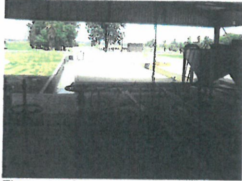
Figure 4 – Grit removal not taking place
