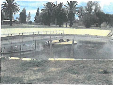
Figure 3 – Primary settling tank
